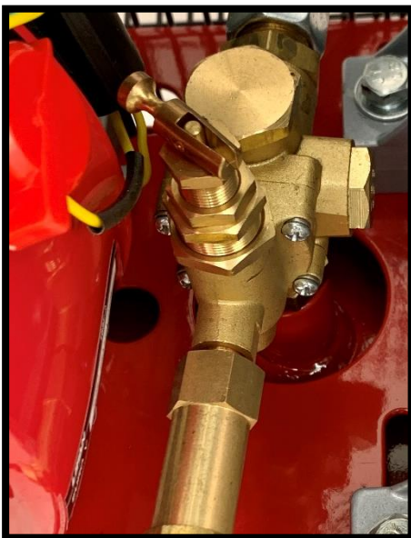
UP – Bypass NEW PIC
